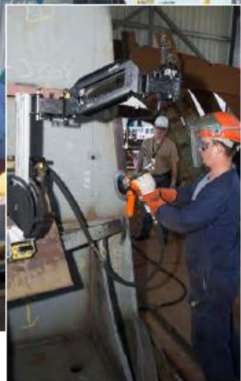
Inset: Joe Thomas , a grinder working on the Ralph Johnson (DDG 114) sonar dome, uses the Equipois zeroG Arm to demonstrate how it helps ease his work. John Forte , project manager with the office of Naval Research, demonstrated the new technology to several engineers and craft leaders.
