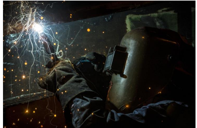
Mechanized and/or automated processes will reduce labor and improve quality during hull fabrication. Ingalls photo
