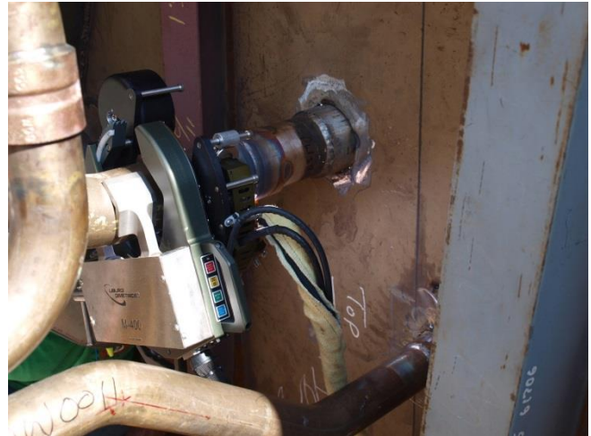
The automation/mechanization of pipe fabrication processes for shipboard applications will improve quality and reduce costs on multiple naval platforms. Ingalls photo
